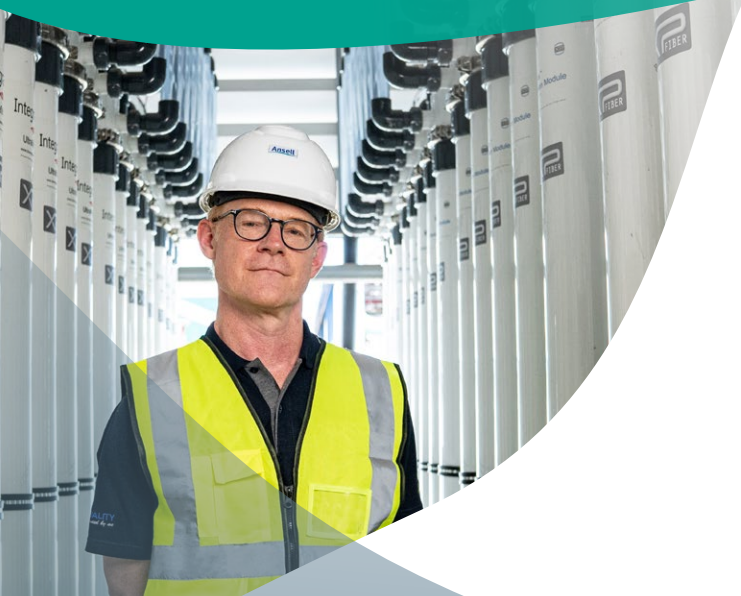
Behind Neil is our reverse osmosis facility, installed at our Thailand plant.
